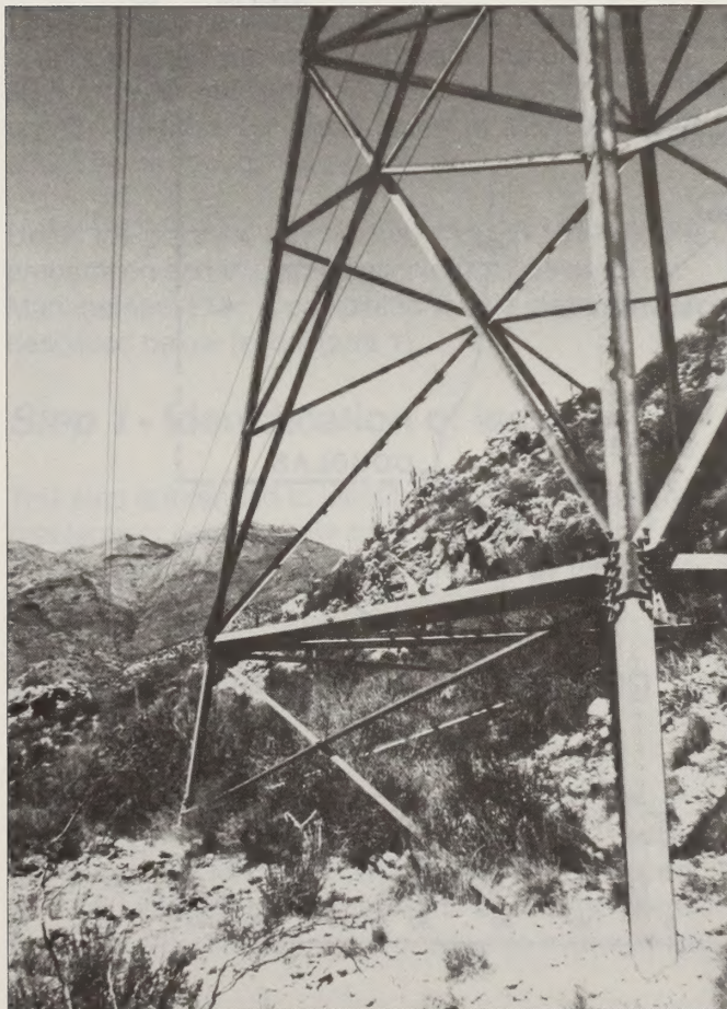
High voltage power lines carrying electricity across public lands.
